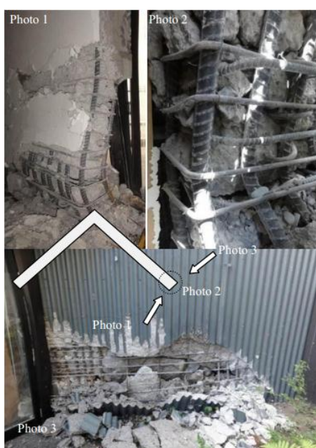
Figure 1 Local buckling damage of a RCSW in a seven-storey building during the 2011 New Zealand Earthquake. (Kam, Pampanin, & Elwood, 2011)
